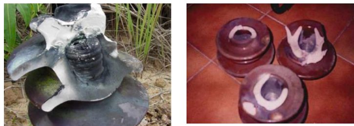
Gambar 3. Isolator pecah akibat flashover [8]
